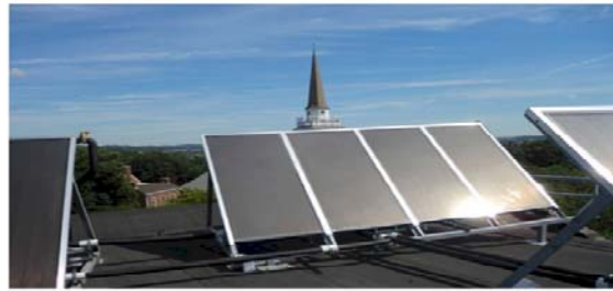
"The curtain-wall-type collectors installed in regular racks; the rooftop installation at Chatham University in Pittsburgh"
