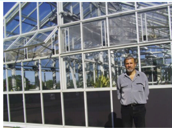
"John Swift, of Solar Tomorrow, shows off the curtain-wall-type solar thermal collectors installed at the research greenhouse at Chatham University in Pittsburgh."
